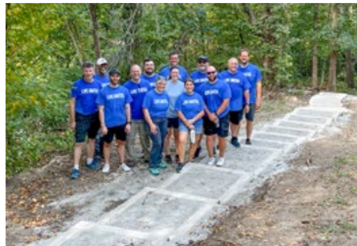
Employees from Ames-based software company, Vertex, stand proudly after completing a trails project at McFarland Park as part of the United Way's Day of Caring on September 13. The volunteers hauled gravel to fill a newly-built set of trail stairs.
